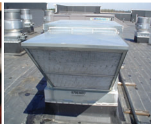
Improperly flashed rooftop ventilator
