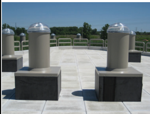
Over 20 photo tubes were installed in the roof to bring natural light into the building interior.
