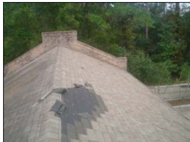
Damaged shingle roof Baton Rouge, LA
